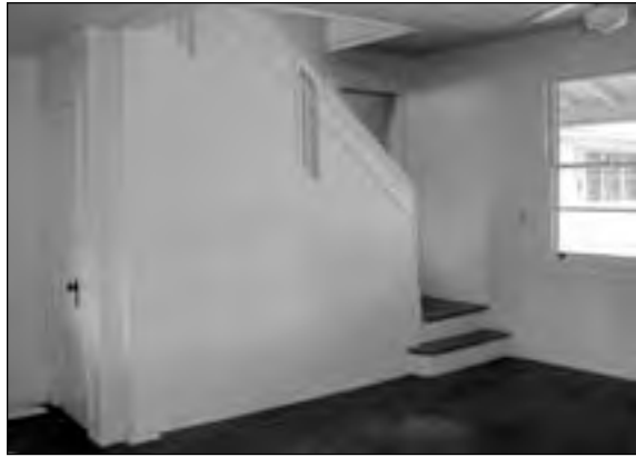
World War II Company Officers' Apartment living room and stairway Source: Mason Architects, Inc.
