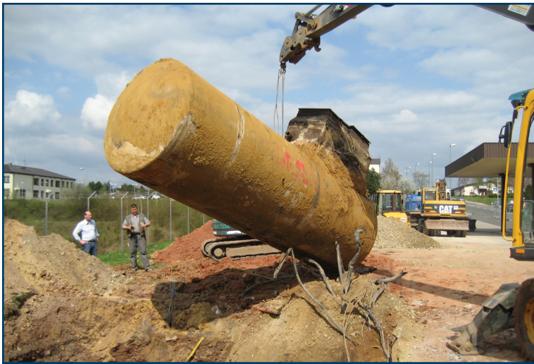
Along with OWS decommissioning, decommissioning fuel tanks reduces maintenance and inspection costs. Removing unused fuel tanks eliminates high risk environmental aspects. It also enables minimal contamination goals to be met.
