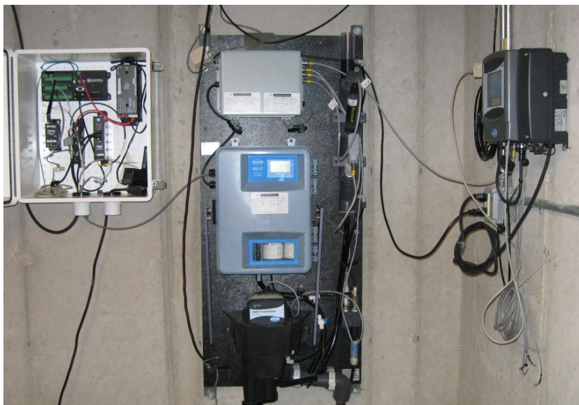
One of three water monitoring panels used to track real-time water pressure and water quality parameters.
