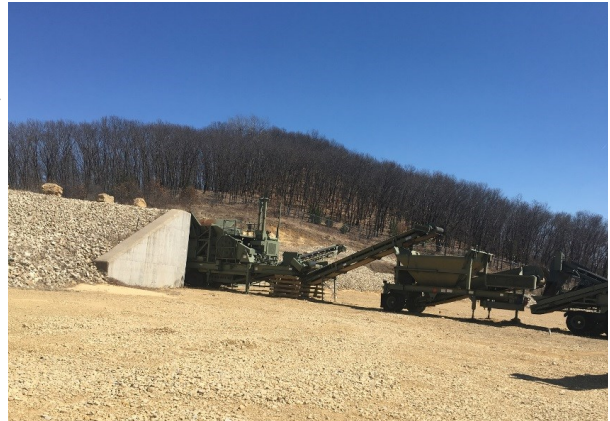
Rock crusher activities at Fort McCoy during an air emission compliance study. The installation undertook this air compliance assessment and air emissions inventory in fiscal year 2018 for all industrial facilities to ensure compliance with air emissions regulations statewide, particularly focusing on emissions from generators.
