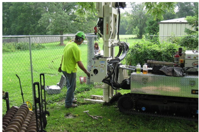
Pictured here, staff install a groundwater monitoring well at Waupun for site investigation activities. The installation achieved complete closure in May 2018, and personnel eliminated offsite impacts to avoid restrictions on adjacent properties.
