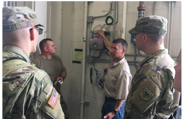
Mr. Scott Rickard, Construction and Facilities Management Office-Environment, trains soldiers to operate a new tank monitoring panel connected to a fueling system. The panel is remotely connected into the Federal network for remote access and efficient management.
