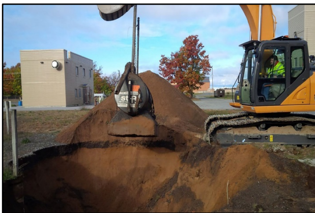
In-house removal of training pit system components at the Fire Training Area.
