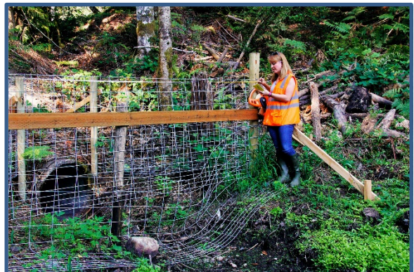
Wildlife biologist inspecting a culvert recently cleared of a beaver dam and debris.
