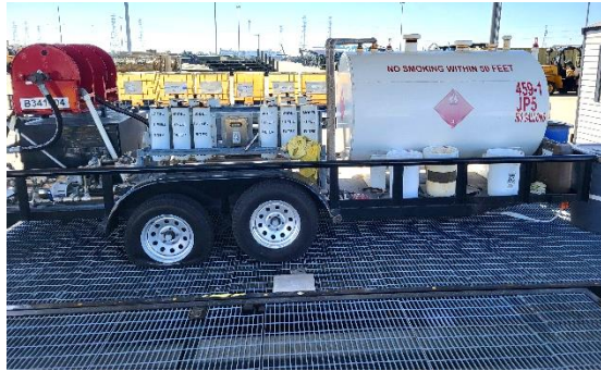
The Fuel Filtration Unit at MCSF-BI, with several off-spec JP-5 totes visible in the background. The FFU can process most off-spec fuel generated at MCSF-BI. However, contaminated fuel cannot be processed through FFU, and is turned in to the MBOS contractor for management as waste.
