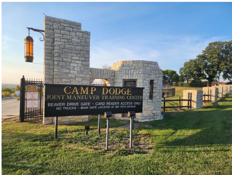
Camp Dodge’s historic stone fence is a landmark for the community and a point of pride for the IAARNG. Restoration of this feature is a major milestone for the Cultural Resources Management program.
