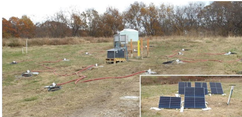
Figure 5. The first ever application of electrokinetic-enhanced bioremediation (EK-bio) for explosives using solar power at LCAAP Area 11. The treatment reduced RDX groundwater contamination over 96% in less than 3-years. This was achieved from problem identification through implementation and confirmation monitoring for a sustainable green remediation approach to optimize restoration timeframes.
