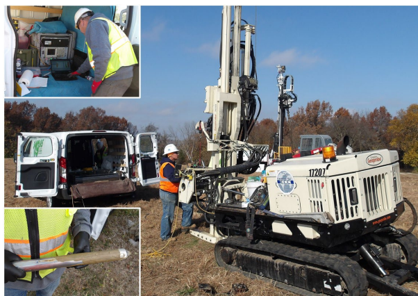
Figure 2. LCAAP conducted a high-resolution site assessment (HRSA) using cutting edge dye-enhanced laser induced fluorescence (DyeLIF) that generated over 103,000 readings to create a precise 3D model of the non-aqueous phase liquid (NAPL) contamination within Area 17B waste pits.
