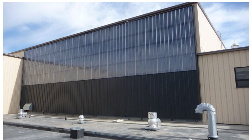
A passive heating solar wall. Energy projects from Energy manager and Planning and Programming efforts are identified through the Operations and Maintenance staff that manage each facility, then depending on cost are completed by that maintenance team for that facility or are passed to the Design and Project Management branch to manage as a typical project.
