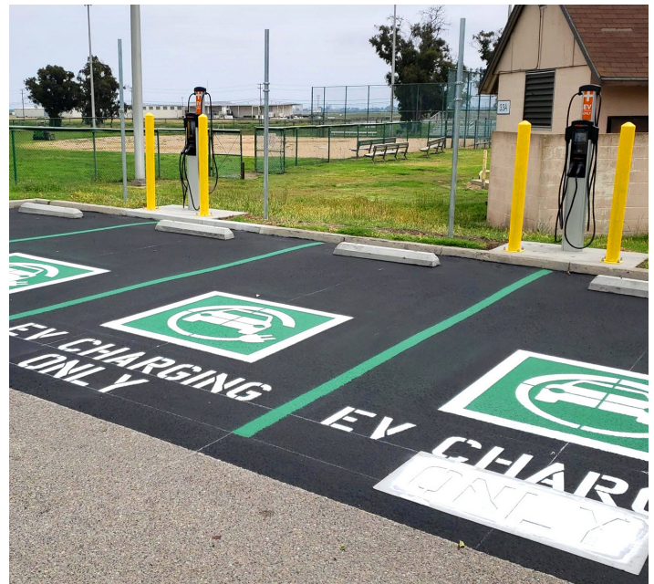
Two Level 2 charging stations for Private Owned Vehicles at the installation's Navy Exchange.
