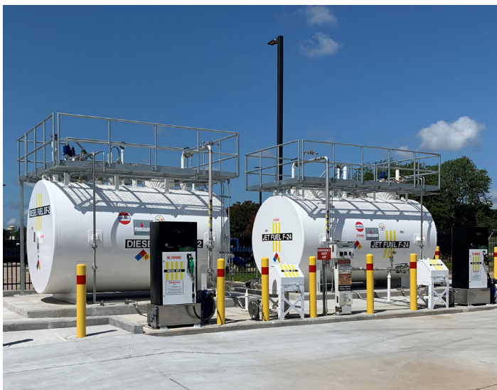
Two newly installed ASTs that replaced three aging USTs in the Aerospace Ground Equipment yard.
