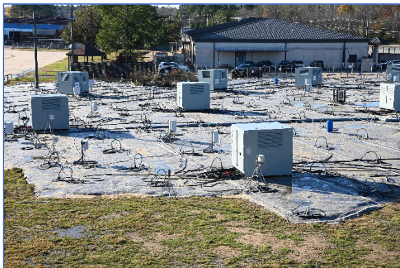
Electrical Resistance Heating System Overhead view of the NTCRA site at Montgomery ANGB.
