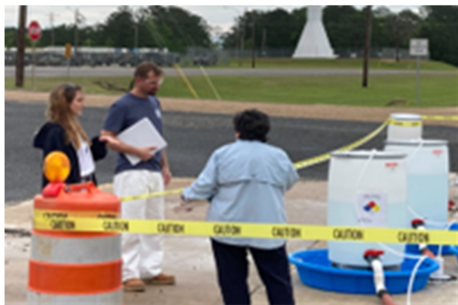
Site inspection of vertical treatment wells around and proximal to exceedance locations installed to deliver material (wash soil) to treat the residual contamination.
