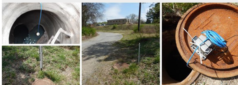
PHOTOS BY WILLIAM COARD, AMERICAN STATES UTILITY SERVICES.
