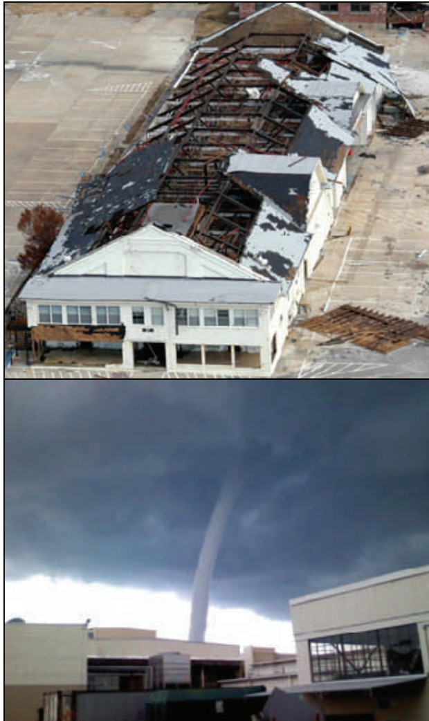
(Photos: Above, Hurricane Ivan damage at NAS Pensacola in 2004. Bottom, a tornado threatens the Landplane Historic District at NAS Jacksonville in 2009. Images courtesy of NAVFAC SE.)
