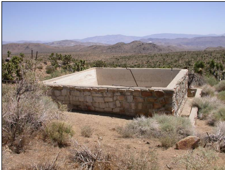
Figure 4-9. Spring reservoir tank constructed by CCC for U.S. Department of Grazing (now BLM), Naval Air Weapons Station (NAWS) China Lake, California
