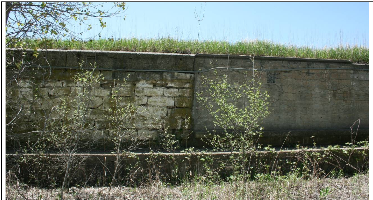
Figure 4-16: Retaining wall in target pit showing transition. Original section at left and WPA addition at right. Note concrete bench at bottom of wall and concrete cap on original section over limestone capstones.
