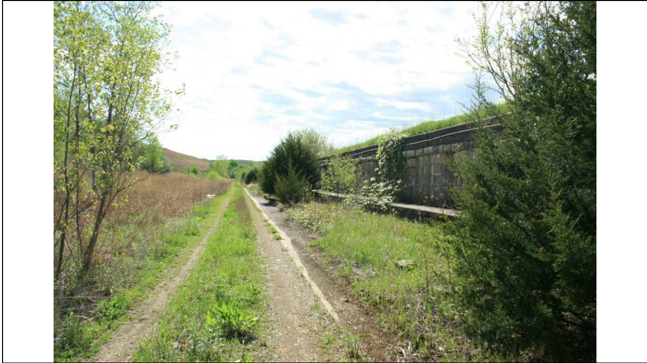
Figure 4-15: Target pit area. Wall and bench at right, concrete gutter at right of two-track dirt road, and hillside at left.
