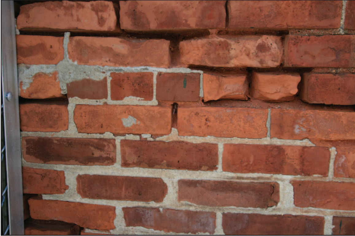
Spalling Resulting from Inappropriate Brick Pointing
