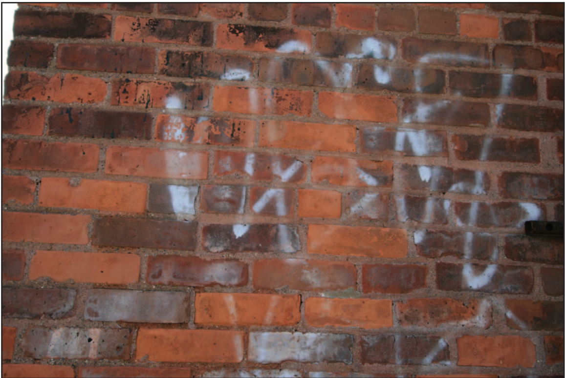
Example of Graffiti Damage
