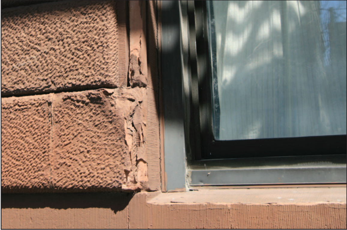
Example of Inappropriate Masonry Repair
