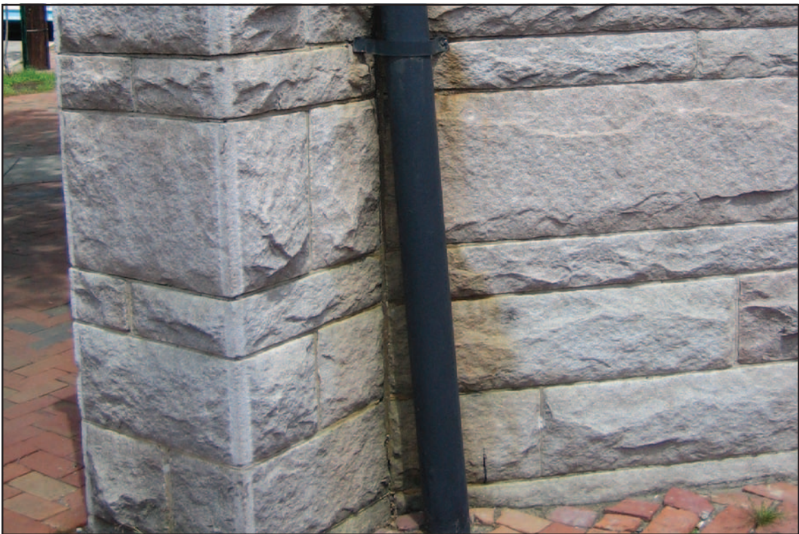
Example of Iron Staining on Exterior Masonry
