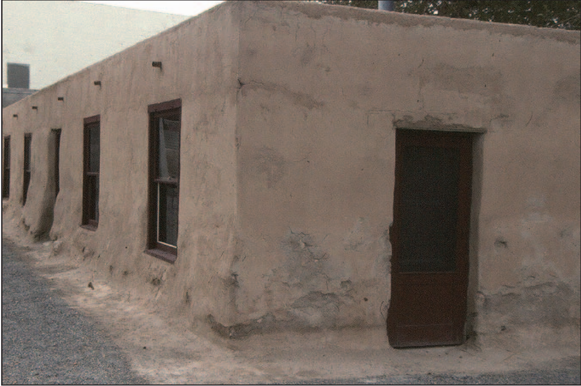
Example of Failing Stucco Application on an Adobe Structure
