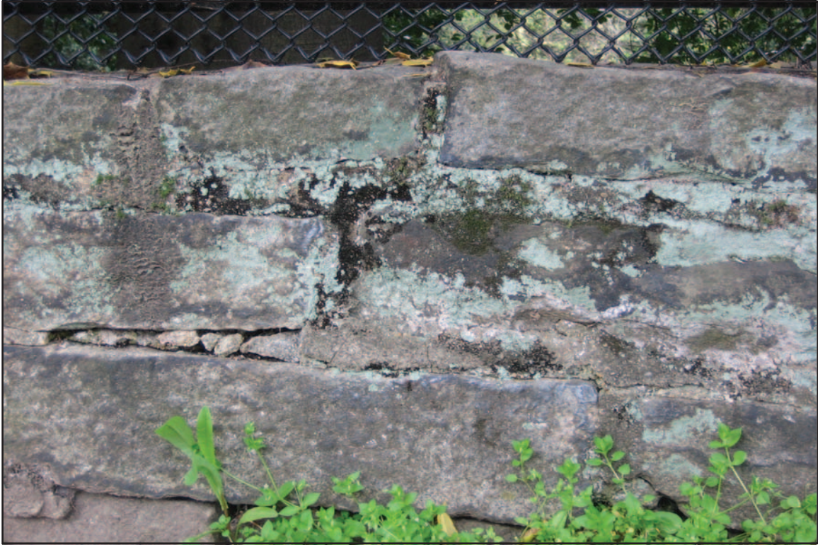
Example of Biogrowth on Exterior Masonry
