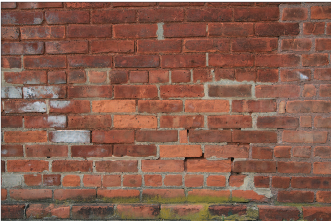
Inappropriate Application of Pointing with Portland Cement Mortars
