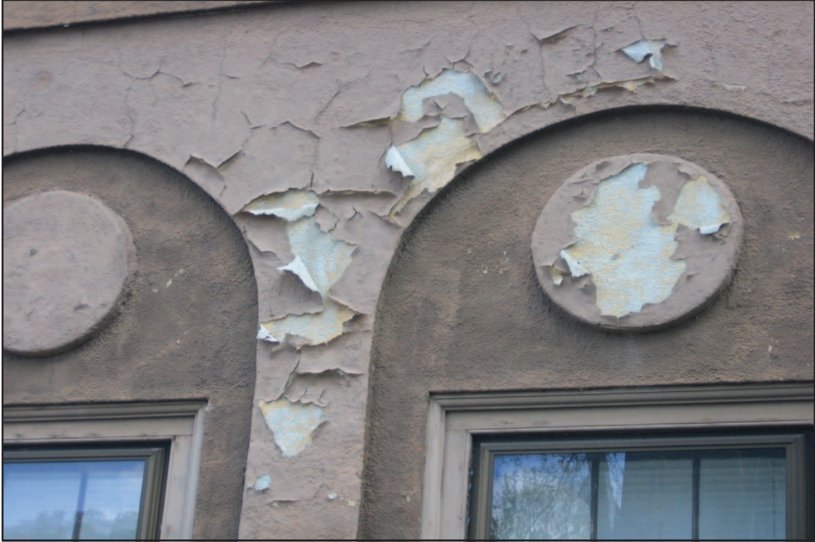
Example of Failed Paint Application on Stucco Exterior
