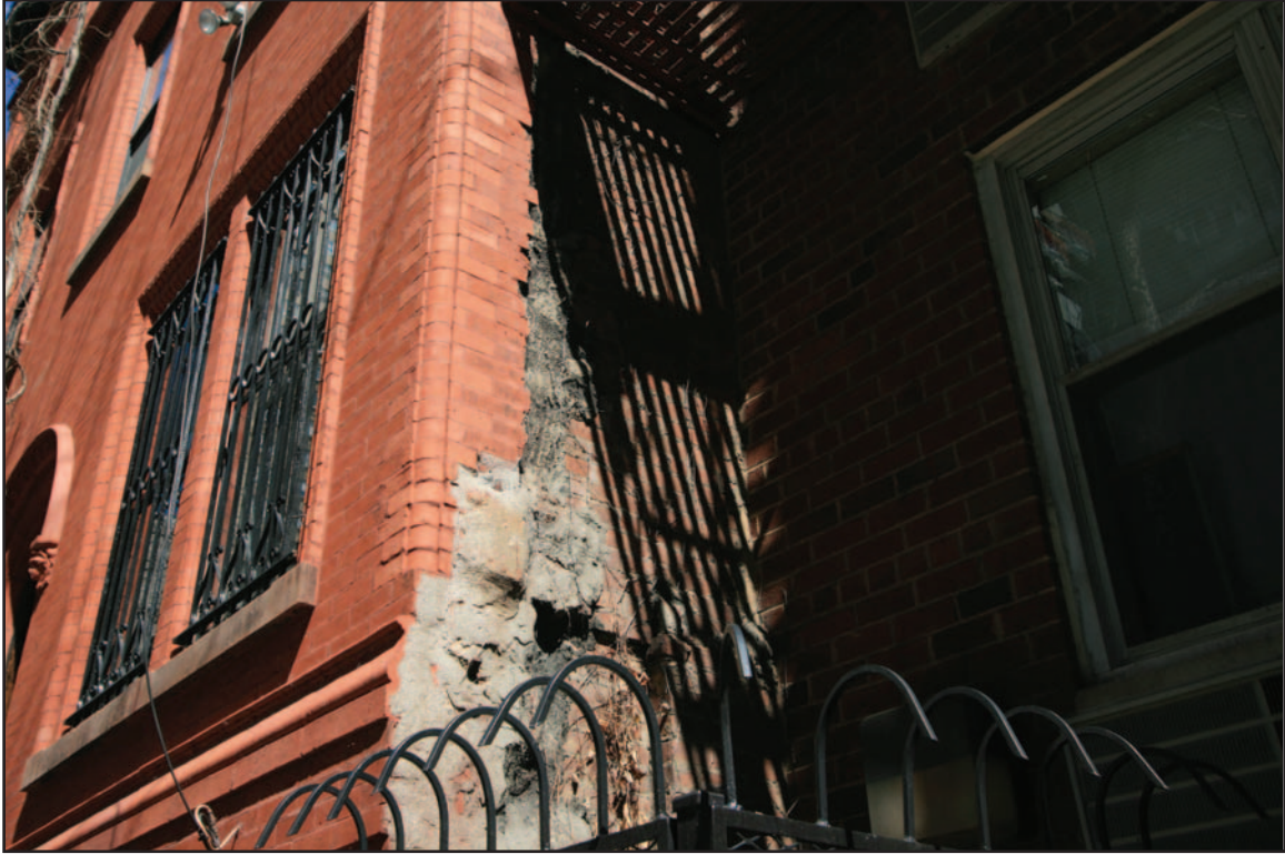
Example of Biogrowth Damage Caused by Creeping Vines
