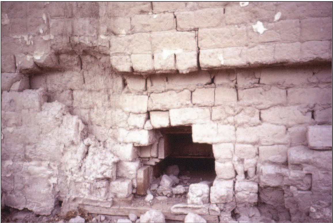
Example of Structural Cracks in an Adobe Structure
