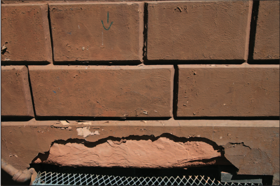
Example of Spalling Brownstone
