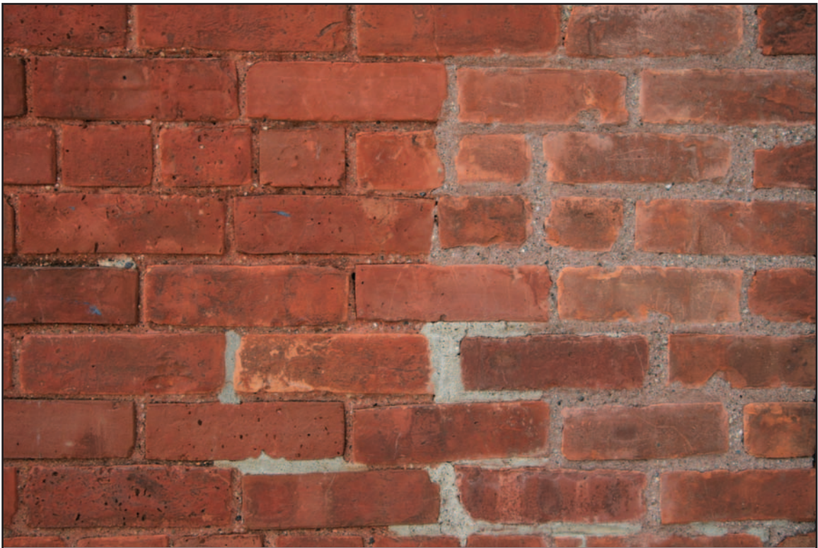
Mismatched Tinted Mortar in Pointing Application
