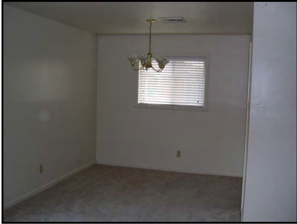
Figure A.2.17. 7541 Talos Drive detail of living room finishes (Capehart housing), NSA Mid-South, Tennessee, 2005. (Photo taken by RCG&A)
