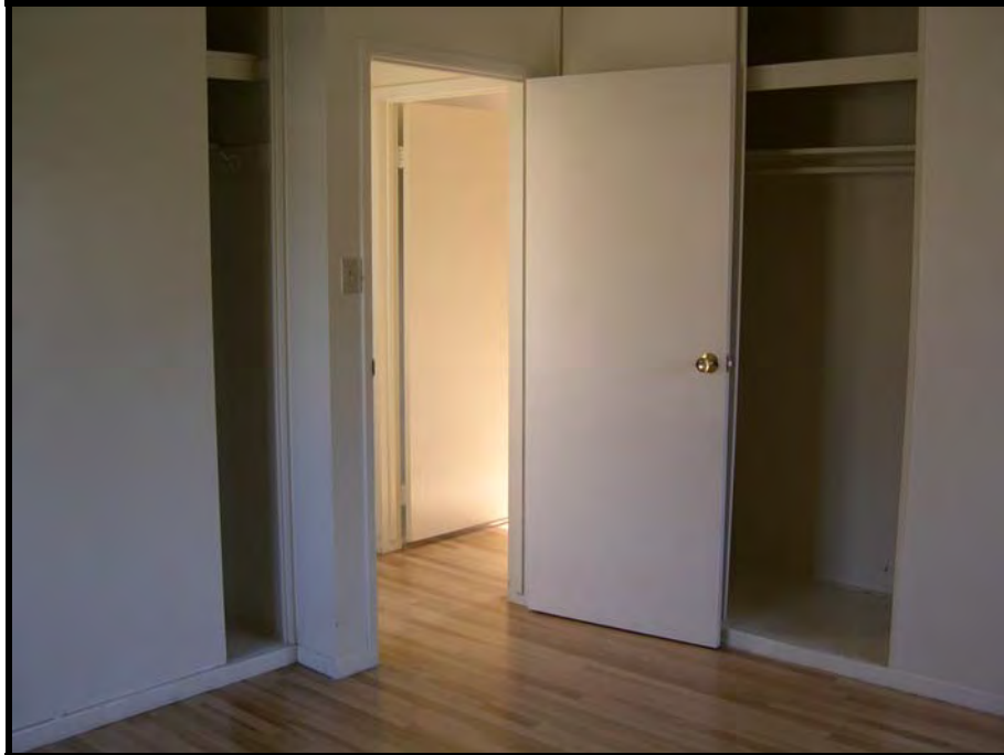
Figure A.5.35. 183 Collins Street master bedroom closets (Type 3M1, New Capehart housing), Travis AFB, California, 2005. (Photo taken by RCG&A)
