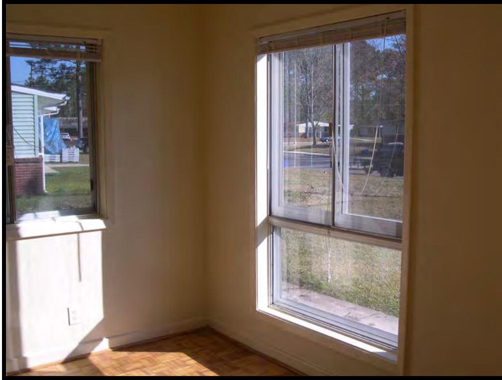
Figure A.3.25. 6 Gates Road (Capehart housing) living room with original window and flooring, MCAS Cherry Point, North Carolina, 2005. (Photo taken by RCG&A)
