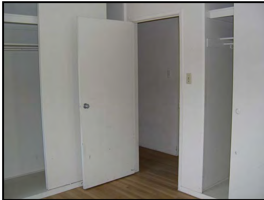
Figure A.5.29. 103 Armstrong Street master bedroom closets (Type 4A1, New Capehart housing), Travis AFB, California, 2005. (Photo taken by RCG&A)
