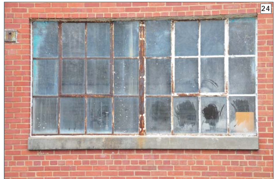
This steel window shows signs of corrosion, a common occurrence in industrial applications. Located at NSF Indian Head, Building 292. (Photographer: Thomas Wright, 2014)
