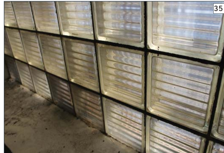
The diffused light and privacy of a glass block panel at NSF Bethesda Building 3. (Photographer: Samantha Driscoll, 2014)
