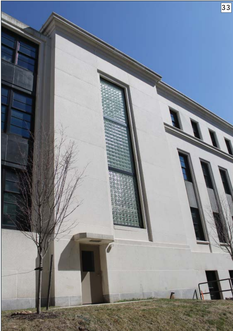
An example of glass block in a stairwell of NSA Bethesda Building 3. (Photographer: Samantha Driscoll, 2014)
