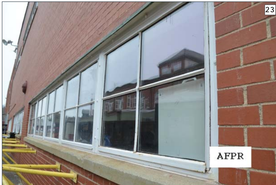
A continuous steel window after rehabilitation at Portsmouth Naval Shipyard, Building 240. (Photographer: Kerry Vautrot, 2014)
