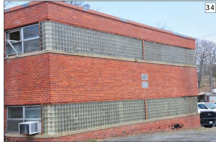
A common application of a large expanse of glass block in a research facility at NSF Indian Head Building 601A. (Photographer: Thomas Wright, 2014)
