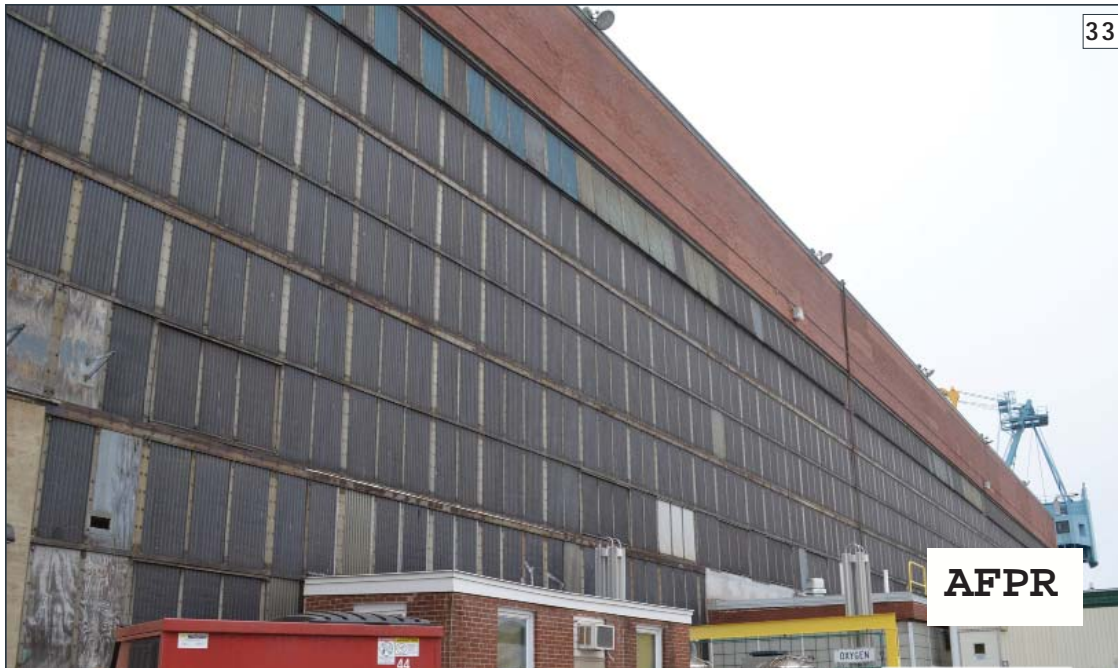
The most common application of corrugated wire glass was in large expanses, shown here in the curtain wall of Portsmouth Naval Shipyard Building 92. (Photographer: Kerry Vautrot, 2014)
