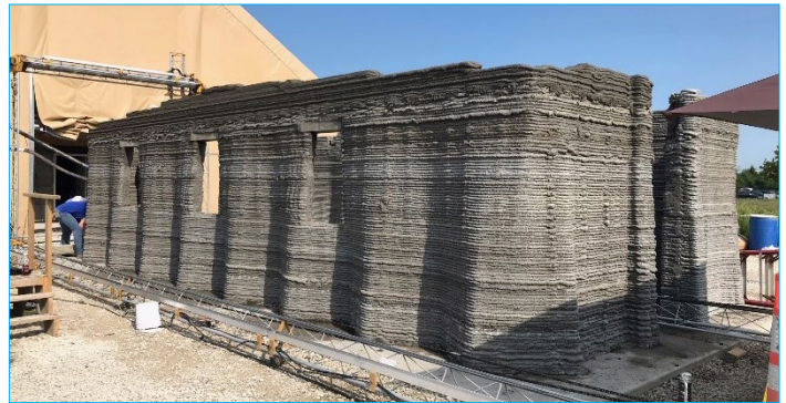
The world's largest concrete 3D printer constructs a 500-square-foot barracks hut at the U.S. Army Engineer Research and Development Center. Source: U.S. Marine Corps
