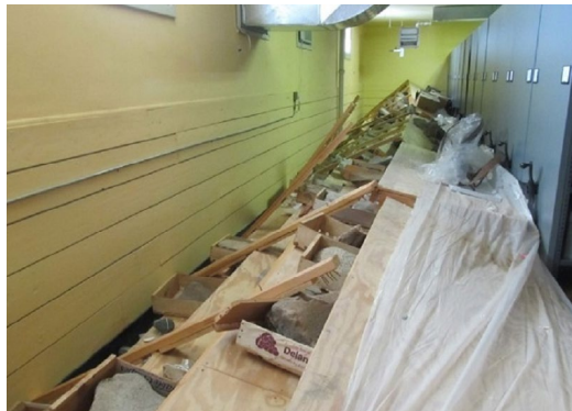
The condition of NAWS China Lake's Curation Facility after the earthquakes of July 4 and 5, 2019. Staff took this photograph during the assessment phase of the earthquake recovery. Source: Secretary of Defense Environmental Awards
