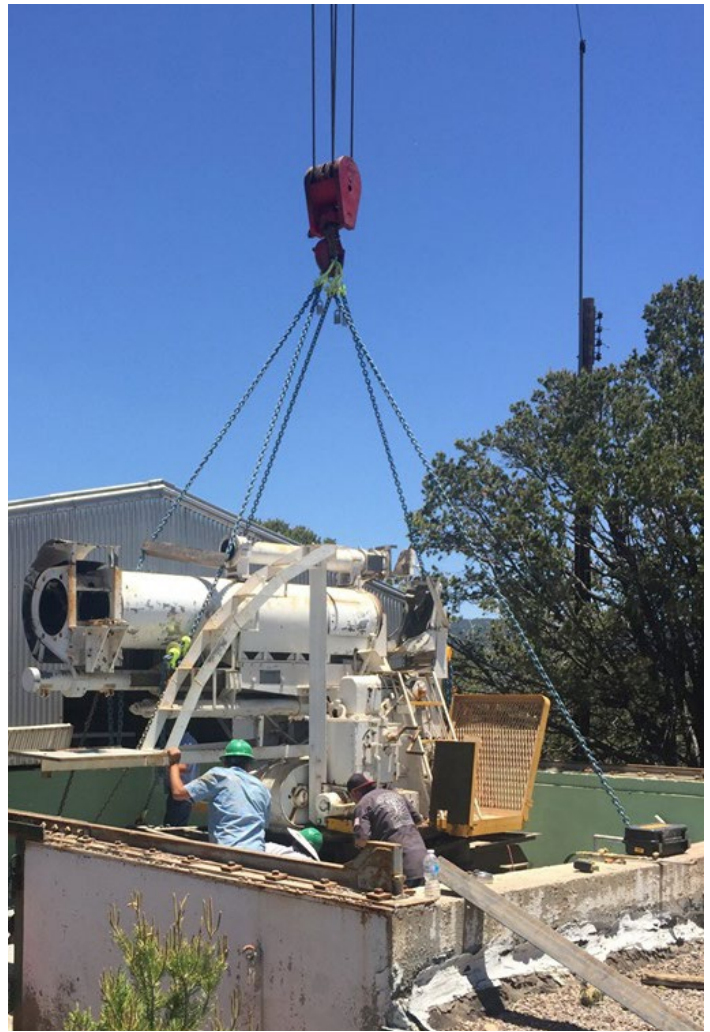
A 75-ton crane extracts Telescope IV from its resting place since 1948. The building roof has been rolled back to expose it, as it is on rails. Source: U.S. Army
