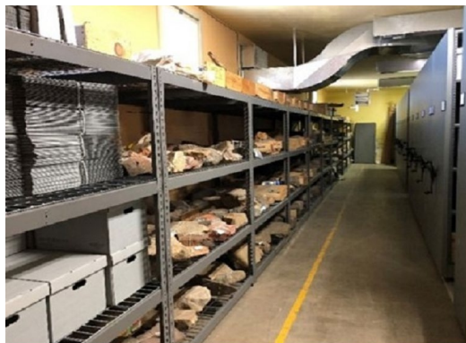
The NAWS China Lake Curation Facility after damage assessment, recovery, and renovation efforts following the earthquakes of July 4 and 5, 2019. Steel reinforced replacement shelving units keep artifacts stable and in place for curation. Source: Secretary of Defense Environmental Awards
