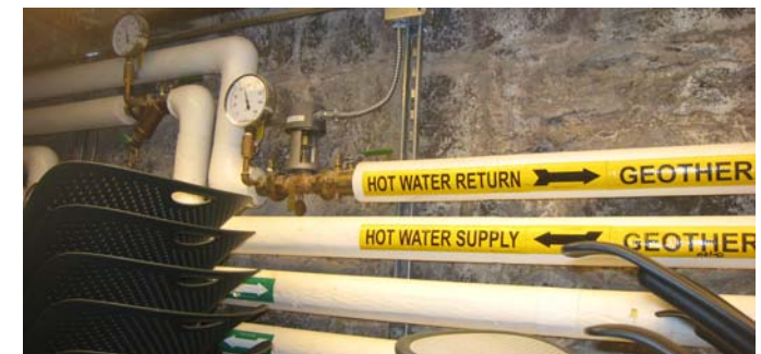
Figure 23 08-15 Geothermal piping in Trinity Church, Boston, MA
