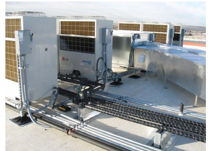
Figure 23 08-9 VRF and Makeup Air Unit on Roof
