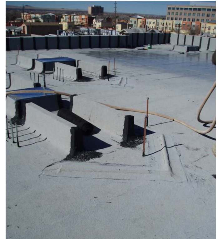
Figure 07 51-1 New insulation and built-up roof applied to historic Coronado School, Albuquerque, New Mexico.
