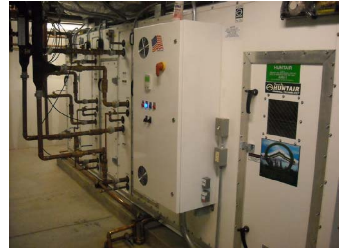
Figure 23 11-12 AHU in a mechanical room AHUs are large pieces of equipment with required clearances. Careful planning is needed if existing mechanical rooms are to be used with newer (often larger) equipment.
