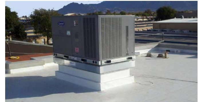
Figure 23 12-2 Packaged Roof Top Unit (RTU) VRF Rooftop Units installed within a screen wall. This is a bird screen to protect the equipment.
