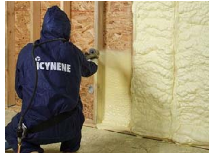
Figure 06 81-11 Notice when the foam is initially sprayed, it is relatively flat, but expands beyond the extent of the studs.
