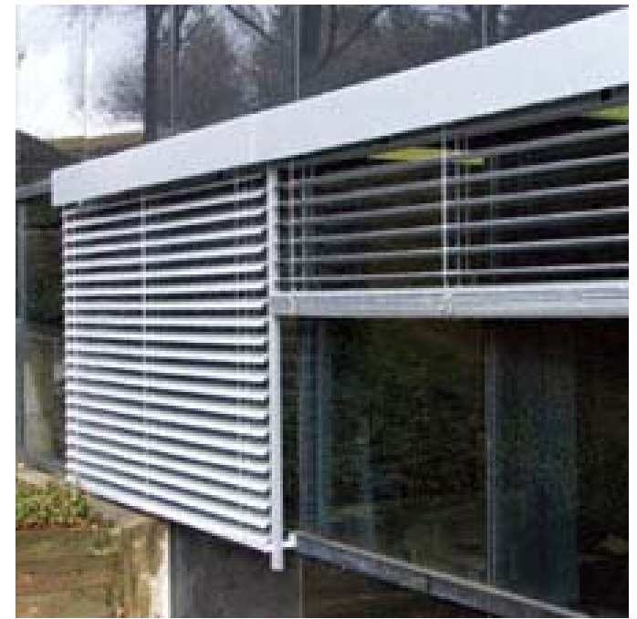
Figure 12 22-4 Exterior Window Blinds
