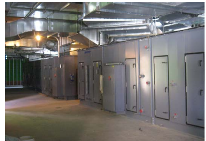
Figure 23 11-13 2 AHU's for a hospital
