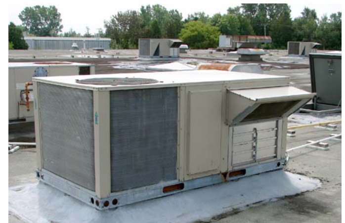
Figure 23 22-8 Rooftop Unit with DX cooling
