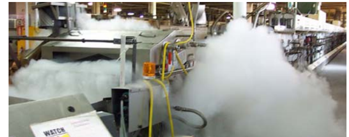
Figure 22 11-15 Clean Agent System
