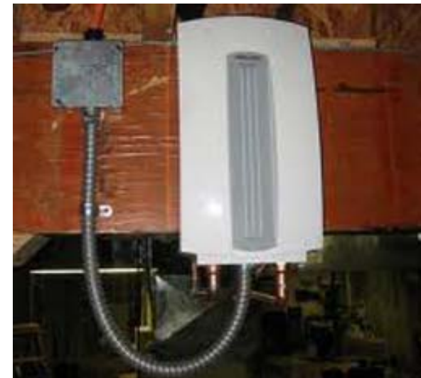
Figure 22 33-25 Mechanical Room electric Tankless Hot Water heater
