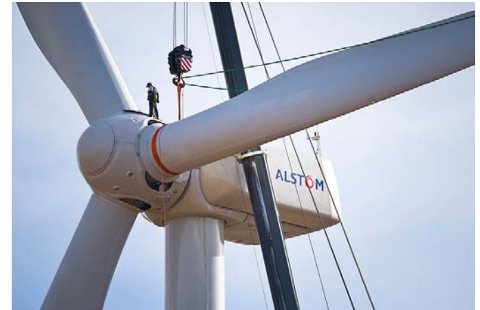
Figure 01 01-9 Large-scale wind turbine
