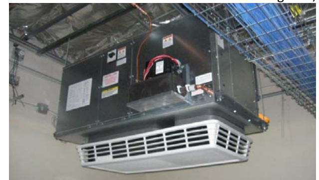
Figure 23 08-13 Interior Split-System Evaporator Coil, For Figures 23 08-11 & 12, see diagram on page 200 for component locations.
