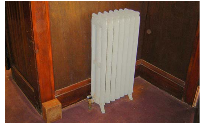
Figure 02 01-17 Radiator at Ft. Stanton
