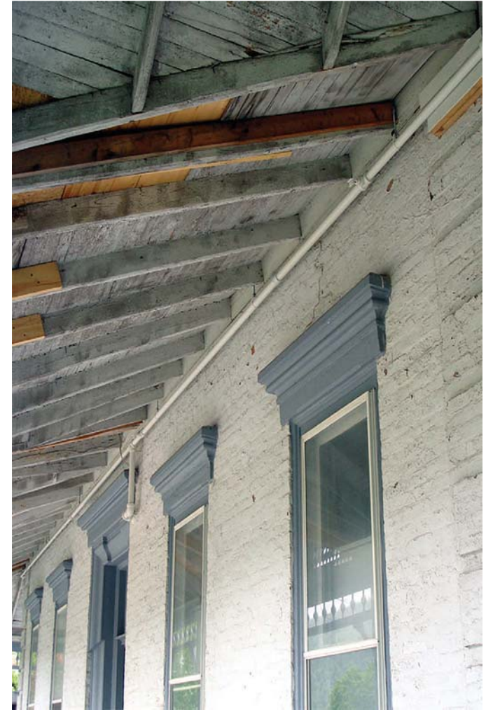
Figure 22 11-5 Dry sprinkler sub-zone on the front porch of a historic building.
