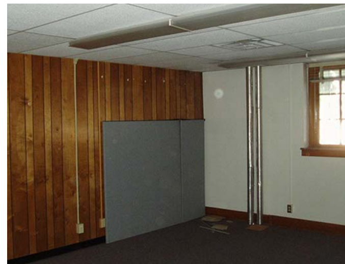
Figure 02 01-23 Before Coronado Elementary School, Albuquerque, NM. Prior to renovation, lay-in ceilings had been installed, and ran into the middle of existing historic windows.
