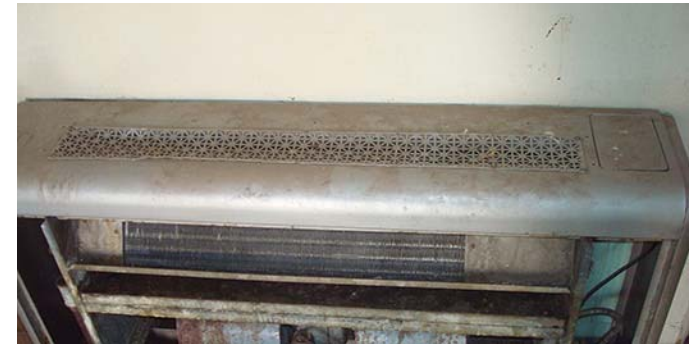
Figure 02 01-15 Decorative radiator cover, from the abandoned De Anza Motor Lodge in Albuquerque, NM, built in 1939.
