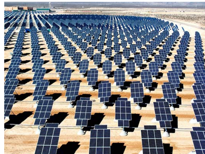
Figure 01 01-1 15MW array on 140 acres of unused land at Nellis AFB. Arrays can be located away from historic districts so as to not disturb the historic character.
