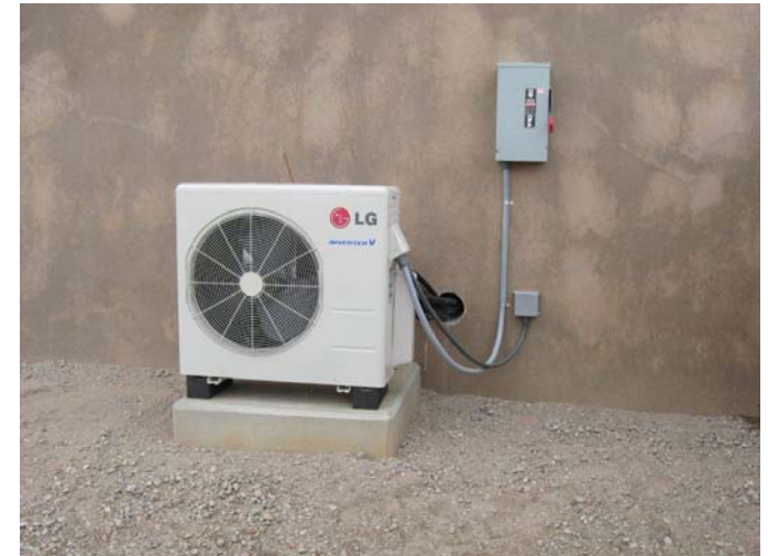
Figure 23 12-8 Exterior condensing unit for a ductless split system (fan visible)
