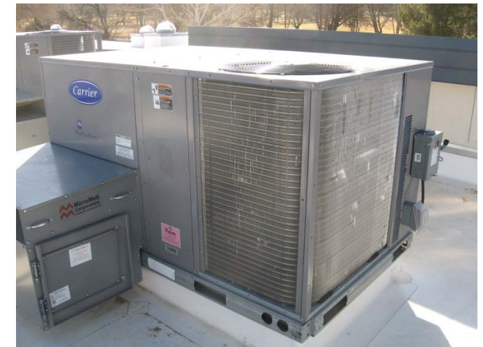
Figure 23 12-3 Packaged Rooftop Unit with Economizer
