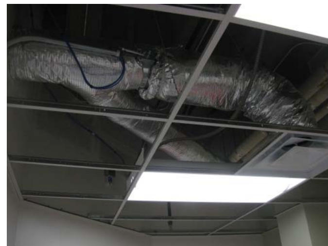
Figure 23 11-16 Insulated ductwork installed above new lay-in ceiling (ceiling tiles not installed yet)
