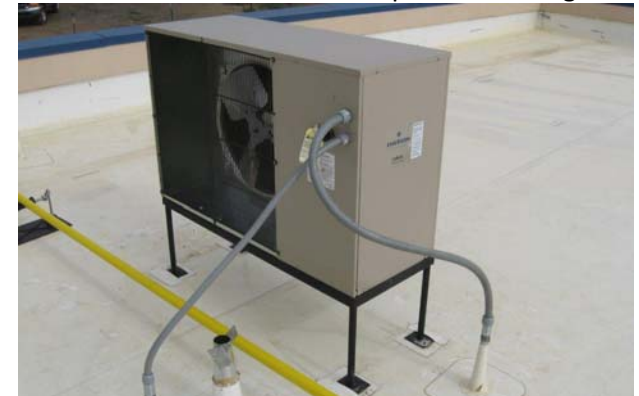
Figure 23 08-12 Roof-Mounted Air Cooled Condensing Unit,
