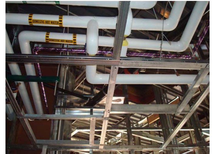
Figure 22 33-18 Overhead, insulated hot water pipes
