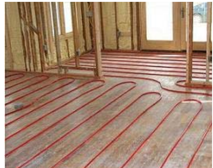
Figure 23 40-6 Radiant Flooring Image from:
