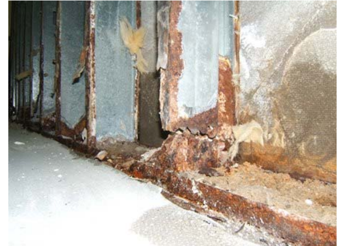
Figure 05 51-1 Rust damage to metal studs
