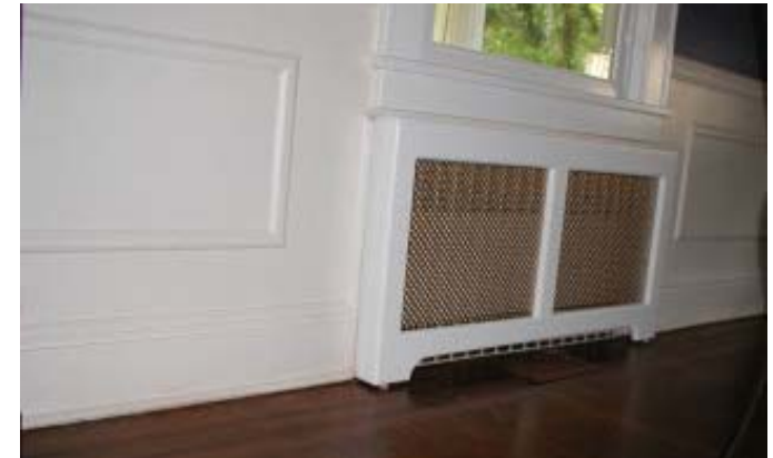
Figure 23 11-6 Radiator furred into the wall
