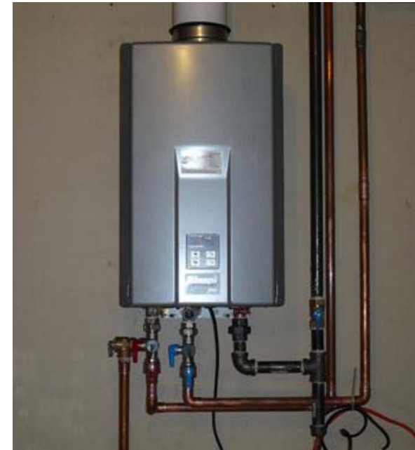
Figure 22 33-24 Mechanical Room gas Tankless Hot Water heater
