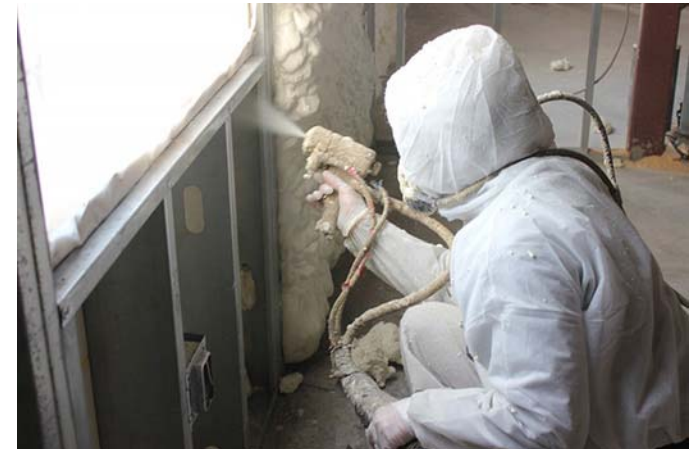
Figure 05 51-9 Notice when the foam is initially sprayed, it is relatively flat, but expands beyond the extent of the studs.
