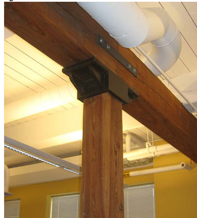
Figure 06 82-4 The wood ceiling was painted white while the columns and beams were exposed and left unpainted. The photos show the integration of modern lighting, HVAC, and fire safety with the historic wood.
