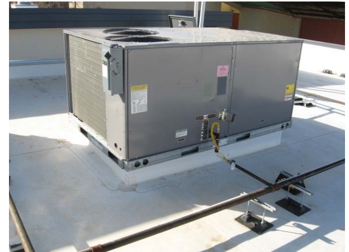
Figure 23 12-4 Packaged Rooftop Unit with Gas Heat
