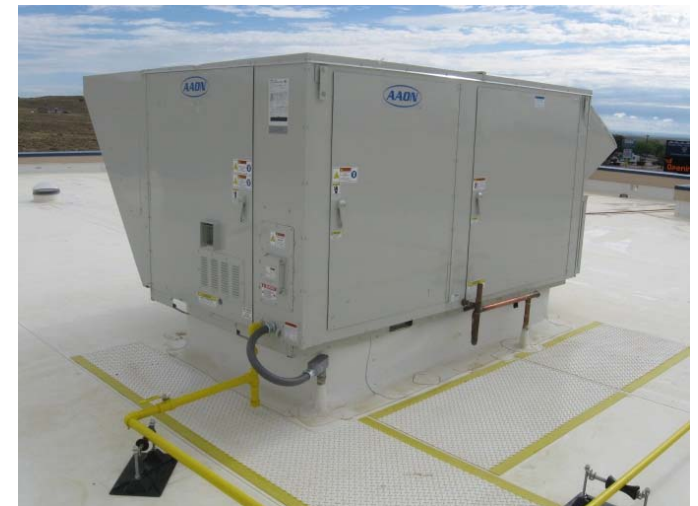
Figure 23 12-5 Variable Air Volume (VAV) Packaged RTU (gas and condensate piping are visible)
