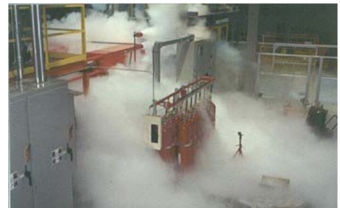
Figure 22 11-16 Clean Agent System,
