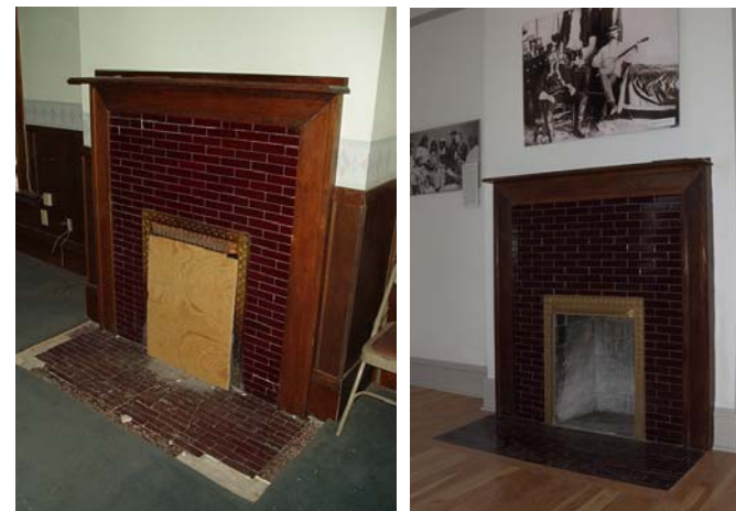
Figure 02 01-8 Before Figure 02 01-9 After Wood burning fireplace at Ft. Stanton, NM. Use as an active fireplace was discontinued.
