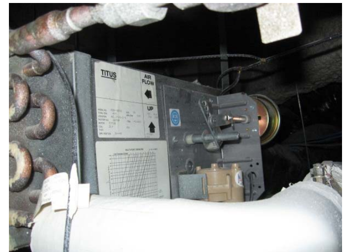
Figure 23 11-11 VAV terminal with Reheat Coil
