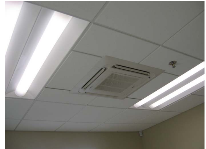
Figure 23 11-8 Installed VRF Fan Coil
