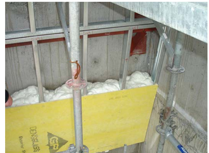
Figure 05 51-10 When installed by an experienced contractor, spray foam can fill and seal around difficult to reach areas.
