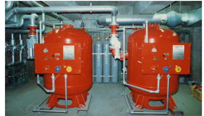
Figure 22 11-14 Dry Chemical Fire Extinguishing System
