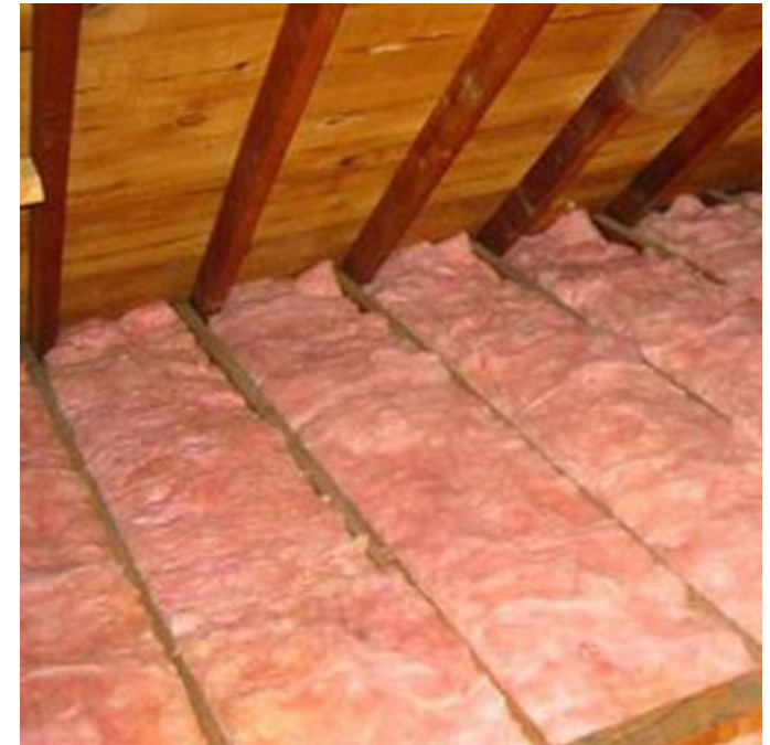
Figure 07 31-4 Fiberglass Batts: Insulation still needs to be added perpendicular to the joists to reduce thermal bridging.
