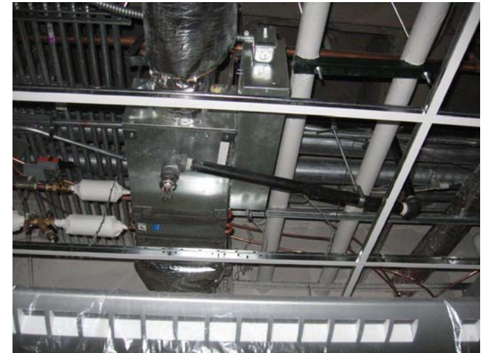
Figure 23 11-10 VAV terminal with Hot Water Coil
