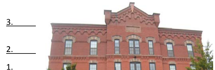
Figure 07 01-1 Numbers reflect different additions and renovations that can be seen in the cornice detailing and brick color.
