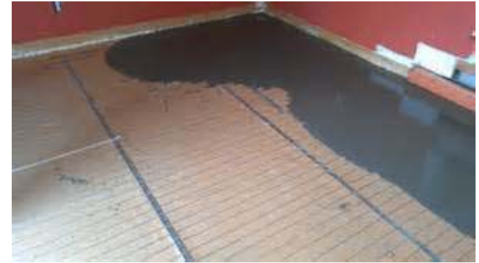
Figure 26 22-4 Electric radiant heating cables being installed in a concrete floor system. SHPO must review and comment on any option that installs a brand new floor.
