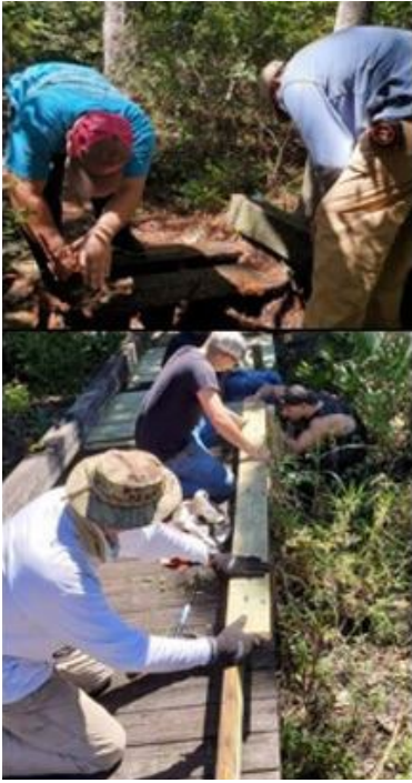
NPLD 2021 volunteers assist with removing garbage and repairing boardwalks at the Grace Brown Nature Trail at Hurlburt Field AFB. Source: NEEF
