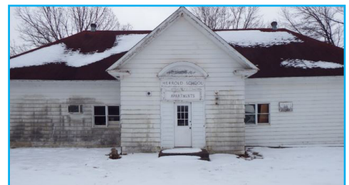
Herrold Schoolhouse in the process of restoration to restore historical features of significance. Source: Secretary of Defense Environmental Awards
