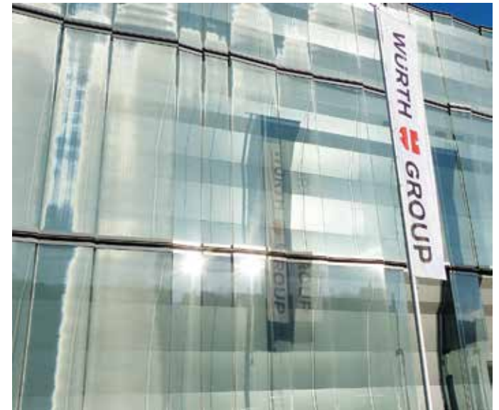
The façade of the WÜRTH Building in Switzerland is mostly glass, laminated with a fabric that is black on the inside but aluminium-coated outside. The inner surface delivers good visibility, and the fabric provides shade and interesting visual effects outside. Preliminary studies by the Swiss Ornithological Institute suggest that the materials used in this building may also deter bird collisions. Photo by Hans Schmid
