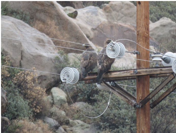
A pair of golden eagles perch on a power pole at WSMR, New Mexico. The two phases closest to the eagles are de-energized. Source: Debbie Nethers
