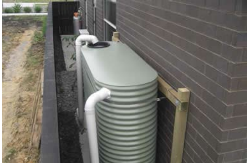
Figure 10. Small-scale, low profile above ground rain collection system ( www.tanksalottx.com ).
