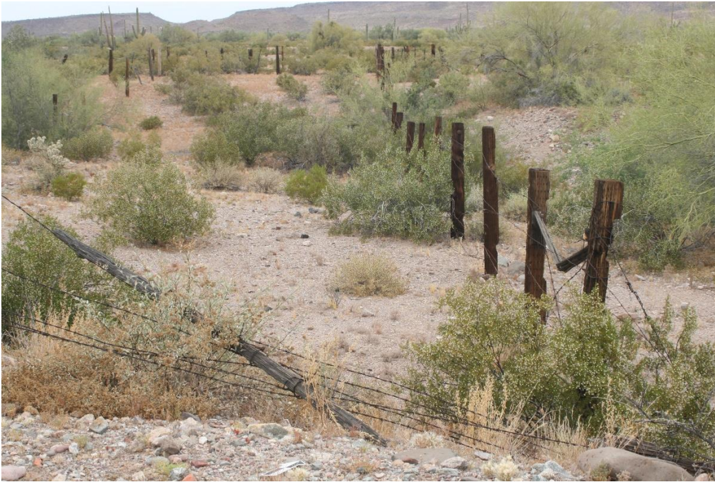
Figure 71. Site AZ Z:6:81 Feature 2 stock corral and chute from the top of Feature 7. View from S to N.
