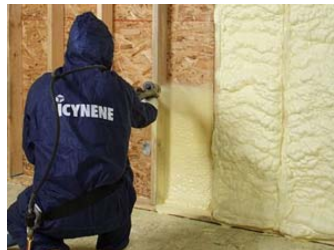
Figure 06 81-11 Notice when the foam is initially sprayed, it is relatively flat, but expands beyond the extent of the studs.
