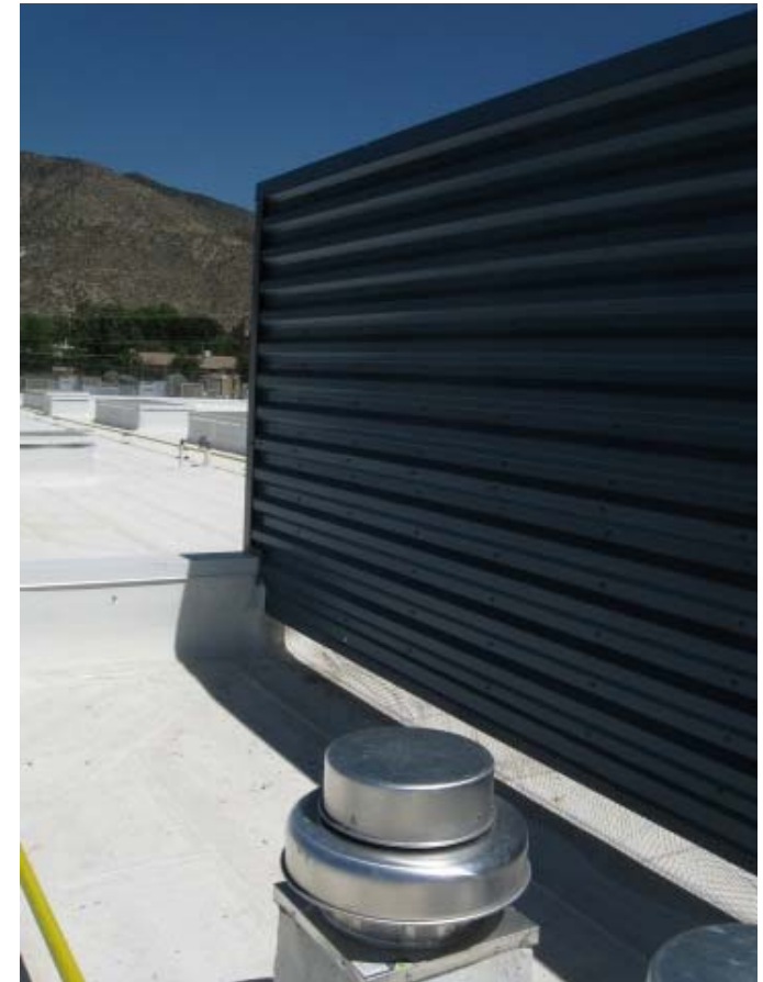
Figure 23 12-1 Rooftop Screen Wall, screens can make the installation of both roof mounted and pad mounted HVAC equipment more acceptable for historic buildings.
