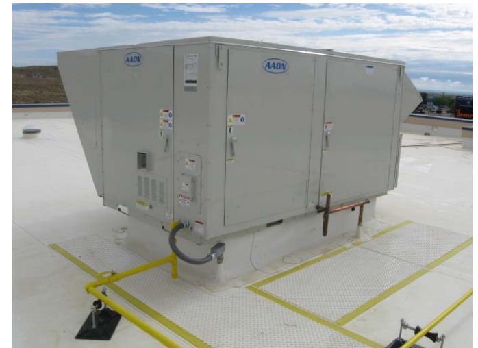
Figure 23 12-5 Variable Air Volume (VAV) Packaged RTU (gas and condensate piping are visible)
