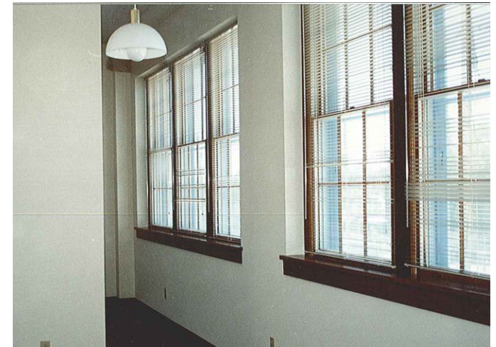
Figure 08 52-2 Installed Back up Windows
