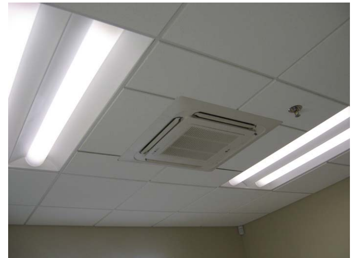
Figure 23 11-8 Installed VRF Fan Coil
