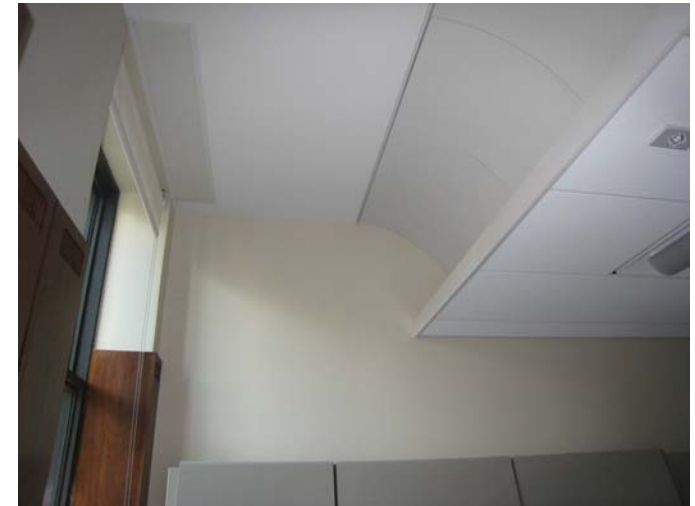
Figure 23 11-15 Ductwork concealed in a new dropped ceiling space, but detailed to respect the historic windows.
