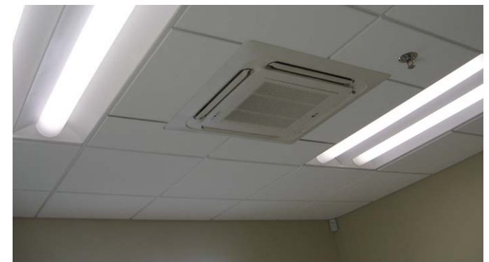
Figure 23 08-8 Installed Fan Coil VRF unit
