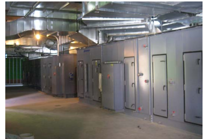
Figure 23 11-13 2 AHU's for a hospital
