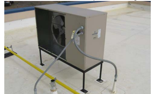
Figure 23 08-12 Roof-Mounted Air Cooled Condensing Unit,
