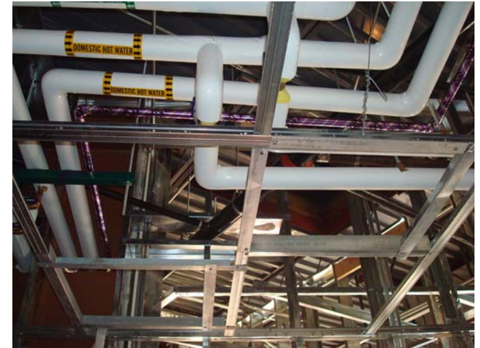
Figure 22 33-2 Overhead, insulated hot water pipes
