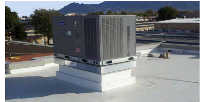
Figure 23 12-2 Packaged Roof Top Unit (RTU) VRF Rooftop Units installed within a screen wall. This is a bird screen to protect the equipment.
