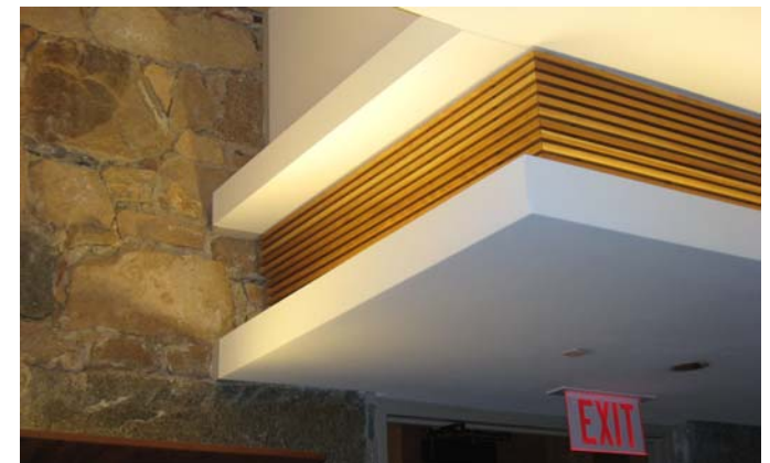
Figure 23 08-17 Supply/return diffuser carefully incorporated into historic fabric of Trinity Church.
