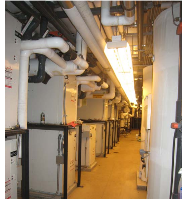
Figure 23 08-16 Heat pumps and blowers at Trinity Church
