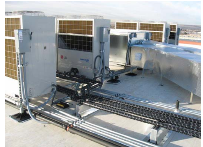
Figure 23 08-9 VRF and Makeup Air Unit on Roof
