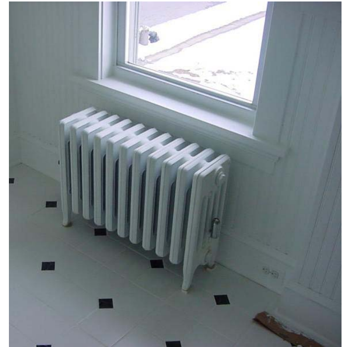
Figure 23 11-3 Radiators are typically located low in the room, like under a window.
