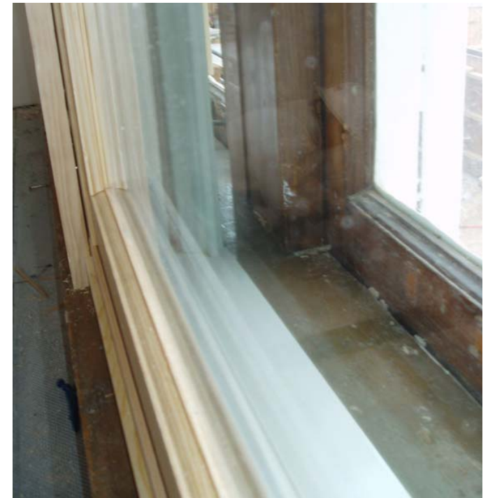
Figure 08 52-3 Close-up of installed interior back-up window
