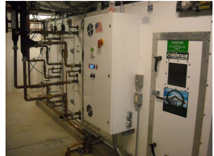
Figure 23 11-12 AHU in a mechanical room AHUs are large pieces of equipment with required clearances. Careful planning is needed if existing mechanical rooms are to be used with newer (often larger) equipment.
