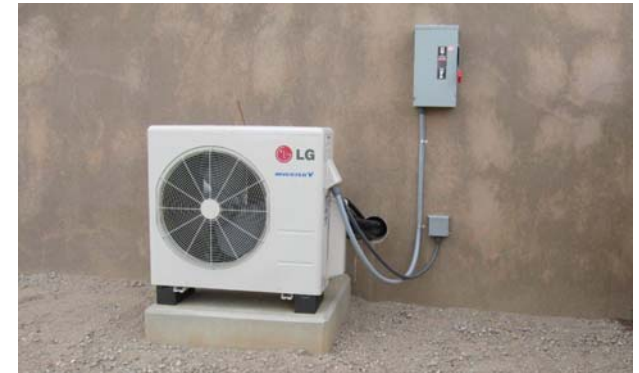
Figure 23 08-11 Pad Mounted Ductless Split Condensing Unit
