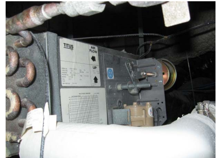
Figure 23 11-11 VAV terminal with Reheat Coil
