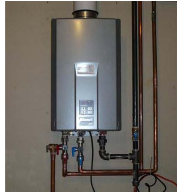
Figure 22 33-8 Mechanical Room gas Tankless Hot Water heater
