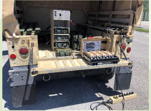
DCPD powering a mobile COC off of vehicle export power at an Initial Technology Insertion at Camp Lejeune
