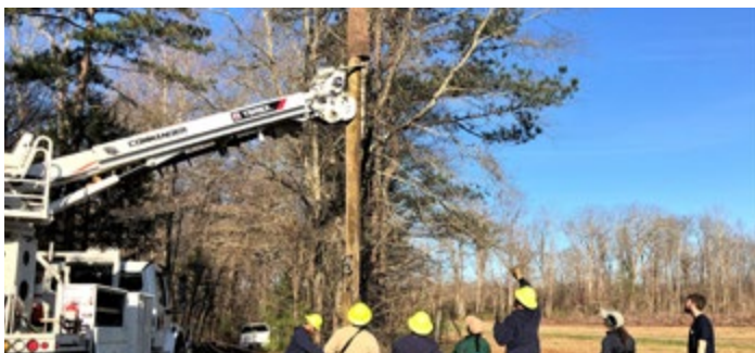
Setting artificial bat roost (Brandenbark) into the ground by Duck River Electric Equipment. The artificial bark is attached to the top of the Utility Pole. In the photo is: USFWS Wildlife Biologist (Leslie Hay), USFWS Volunteers (Jessica Davis and Ben Everett), and Duck River Utility lineman field crew (Sean Scheller, Matt Swan, Eric Burton, and Mitchell Gore). Source: Leslie Hay
