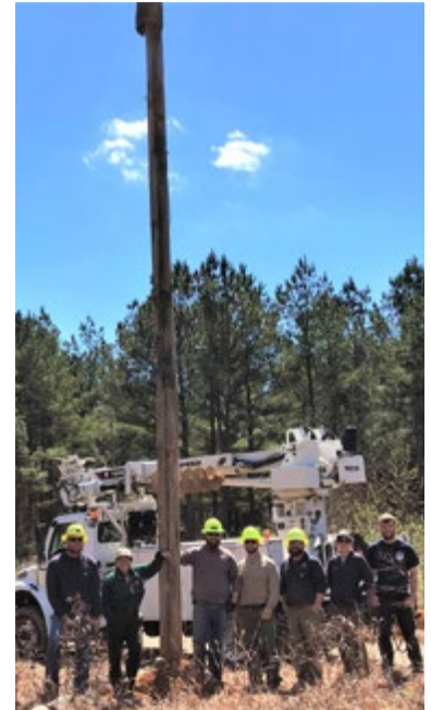
The “build it and they will come” bat project. The artificial bat roost sheet has been attached to the top of the utility pole, which is installed six feet deep into the ground by the utility company equipment. In the picture is: USFWS Biologist (Leslie Hay), USFWS Volunteers (Jessica Davis and Ben Everett), and Duck River Electric Corporation lineman field crew (Sean Scheller, Matt Swan, Eric Burton, and Mitchell Gore). Source: Leslie Hay
