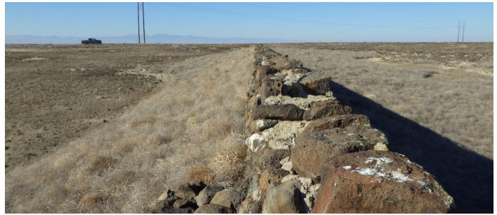
Buildup of hazardous fuels around a historic dam.
